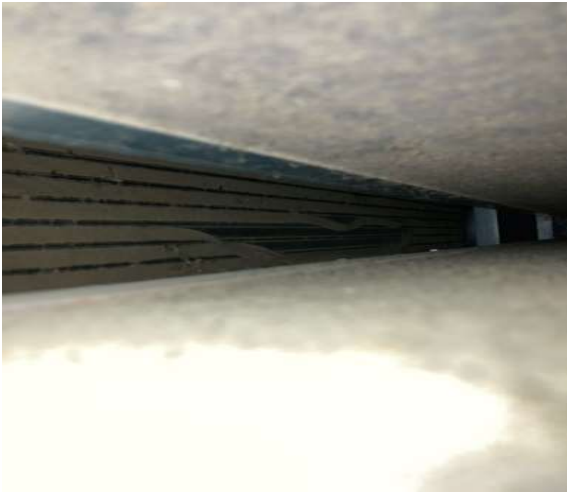
Dust buildup on the oil cooler
