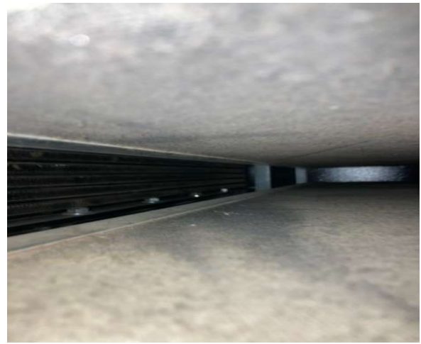
Oil cooler after cleaning
