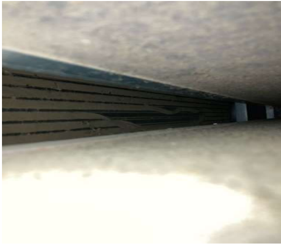
Dust buildup on the oil cooler
