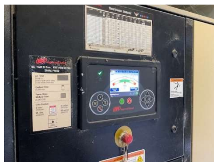
Compressor pressure at 100 psi
