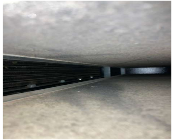
Oil cooler after cleaning
