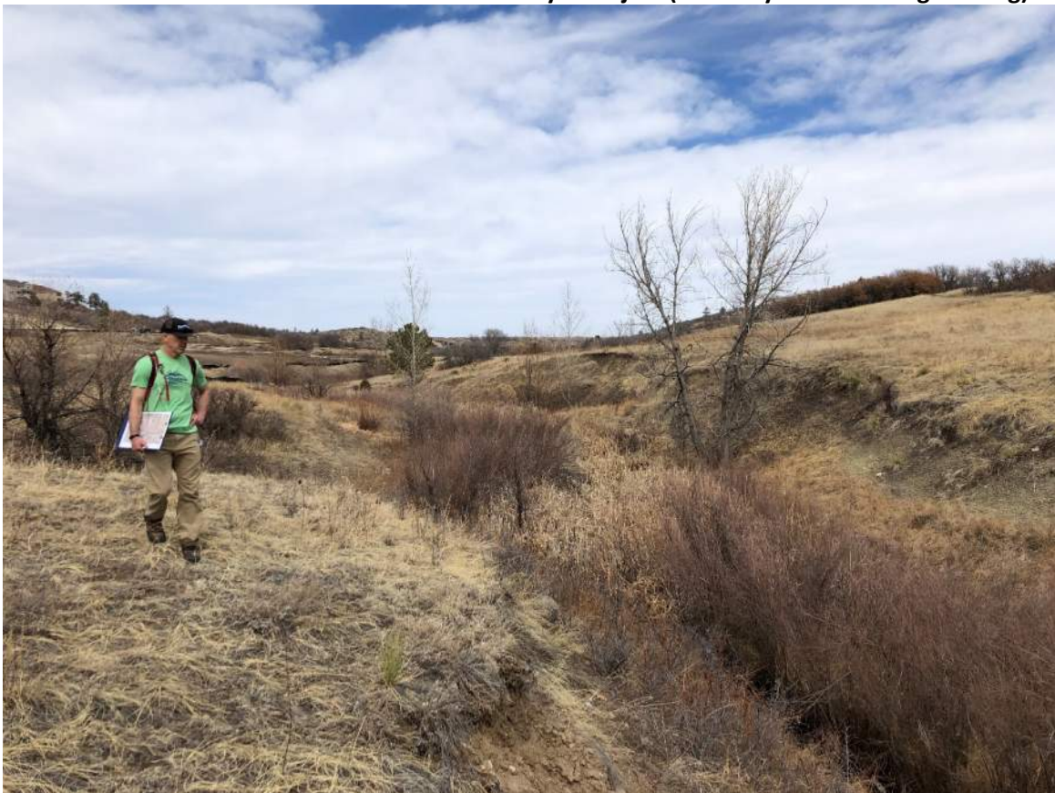
Photo of Bank Erosion on McMurdo Gulch Priority 3 Project (Courtesy of Muller Engineering)
